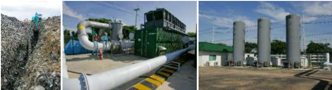
Landfill Gas to Electricity Project (Source: First Climate)
